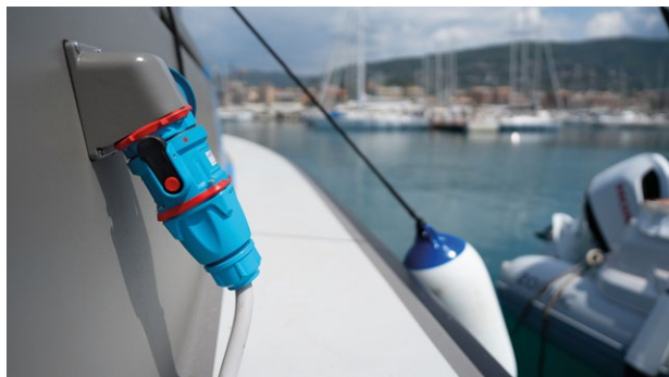
The batteries are charged in the harbour
